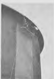
CONTRACTOR'S PAINTERS apply the first of four coats of special paint to a typical round storage tank.
